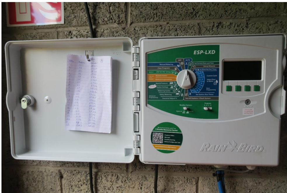
4 – Irrigation controller in pump house
