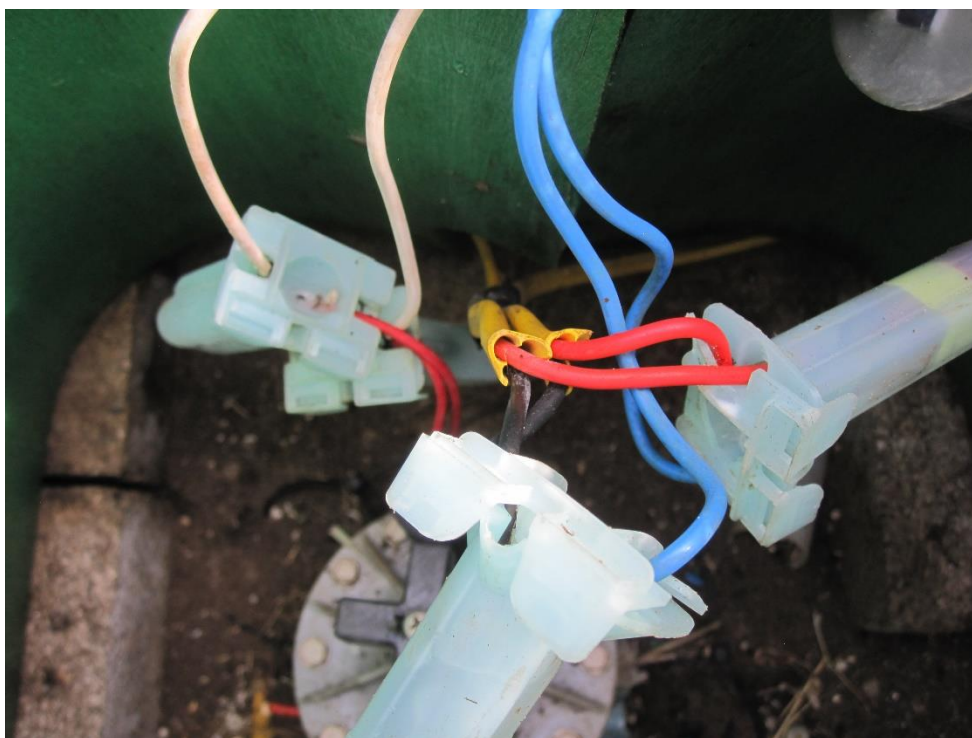
8 – Existing control cable
