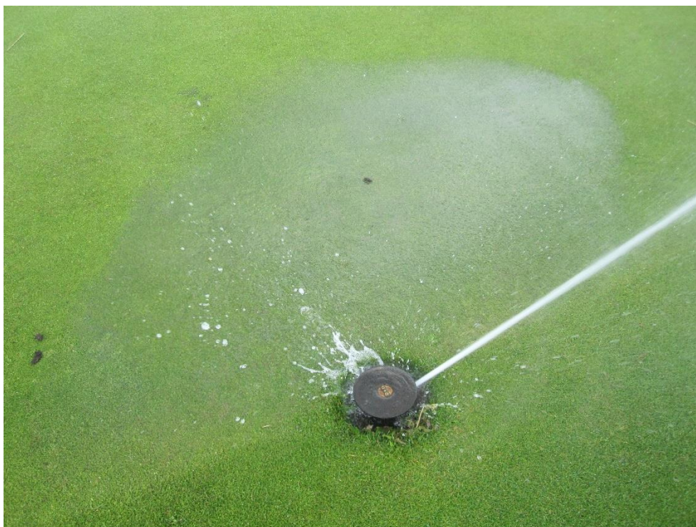
13 – Typical green sprinkler leaking around sprinkler head during operation
