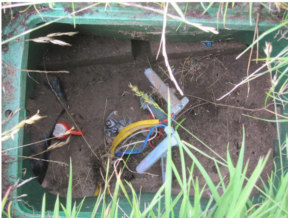
7 – Typical solenoid valve – Note; valve condition and no pressure regulation
