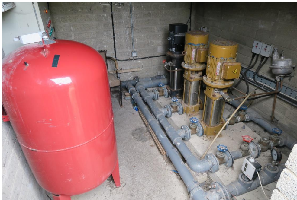
3 – Irrigation pump station within pump house – Note uPVC and manual prime etc
